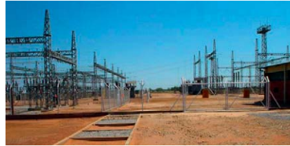
Gerus – high voltage direct current substation, Namibia
